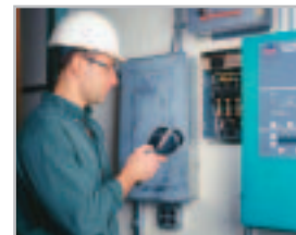
Infrared can accurately and quickly locate faults before failures, shutdowns, or even fires occur.
