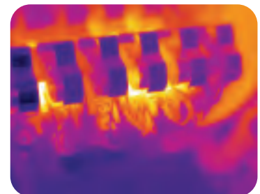
Infrared can accurately and quickly locate faults before failures, shutdowns, or even fires occur.
